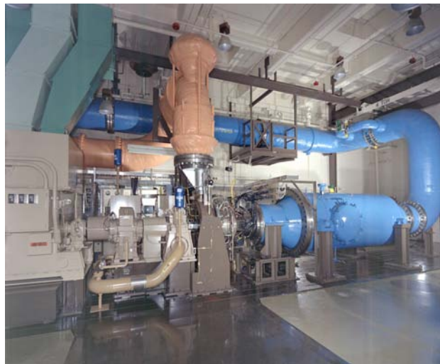
b) Small compressor facility
